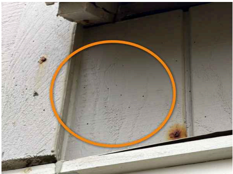
Wood boring beetle exit holes at T1-11 siding
