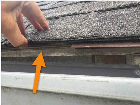
Incomplete/missing drip flashing
