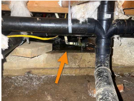
Pooling water under home from significant leakage
