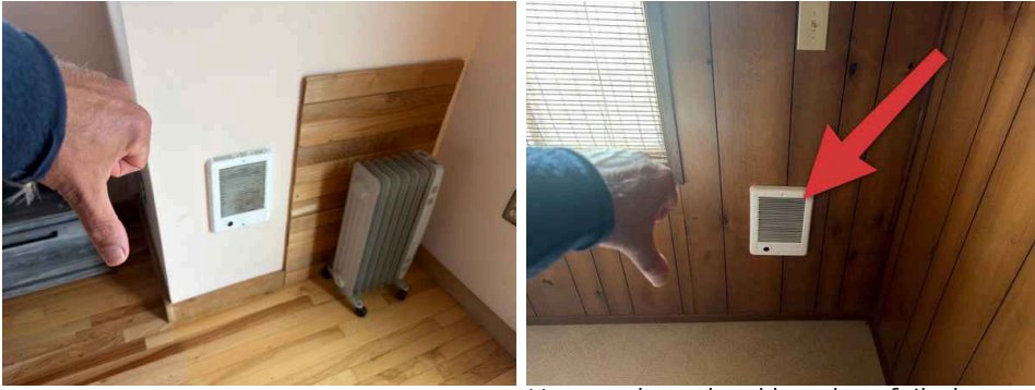
Heater glowed red hot then failed
