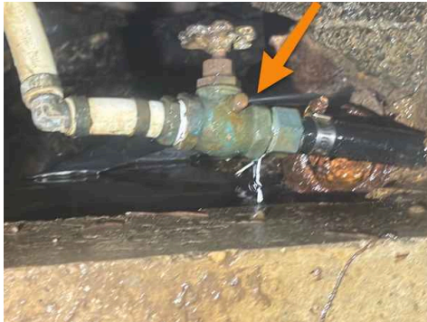
Significant active leakage
