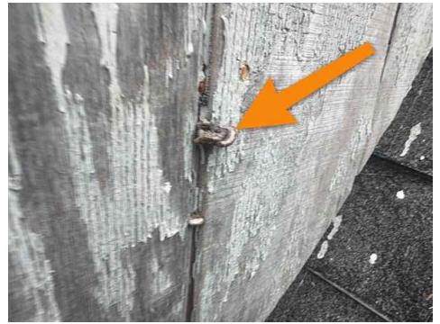
Mushrooms growing out of failed/neglected siding
