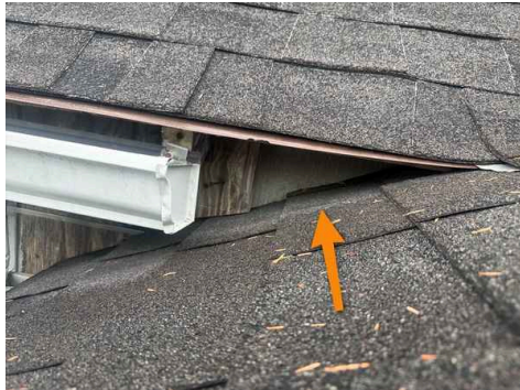
No step flashing
