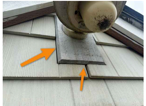
Poor installation: not sealed
