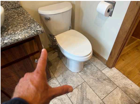
Toilet: loose at floor
